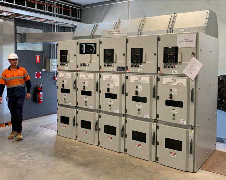
Christies Beach Wastewater Treatment Plant
